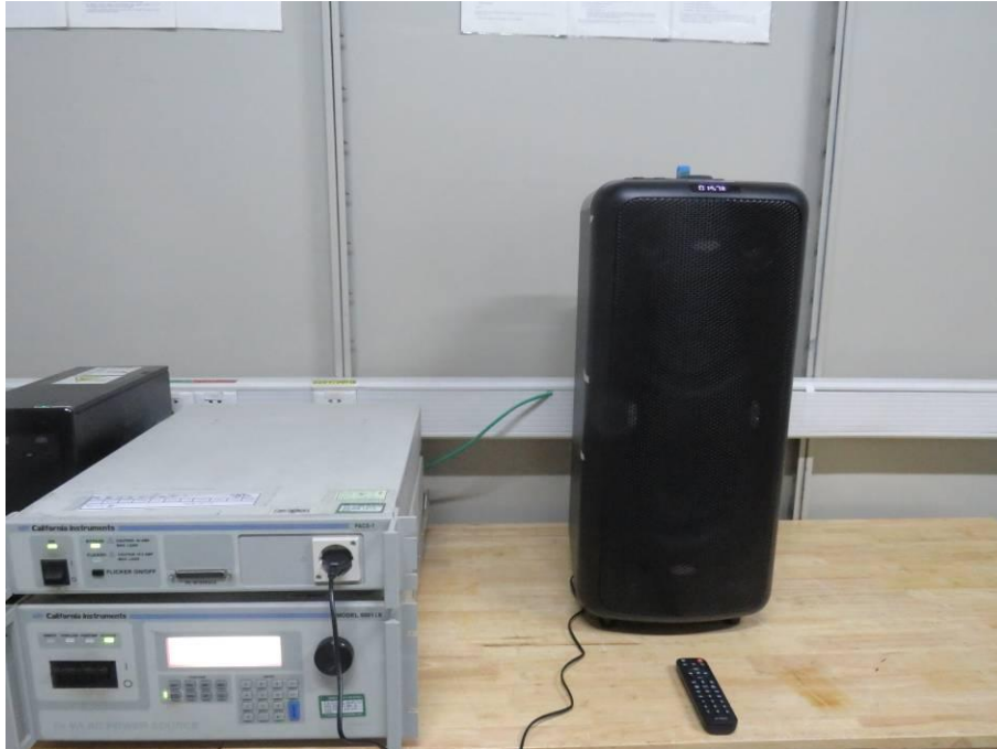
Photo of Harmonic/Flicker Measurement
